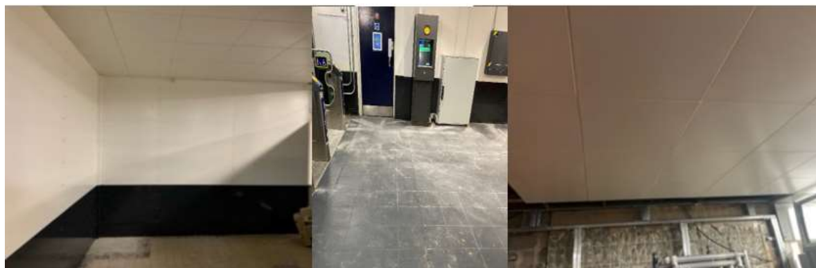
New wall and ceiling cladding and new flooring installed at Finsbury Park Retail Unit
